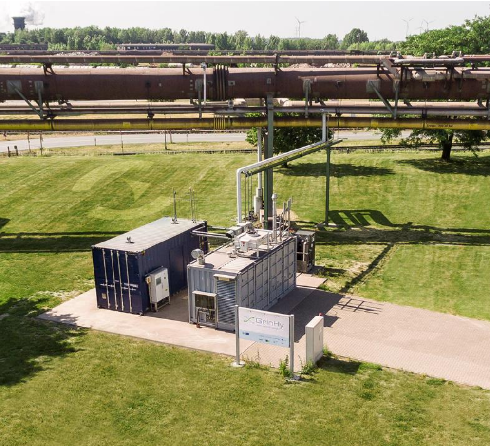
Sunfire Electrolyser installed at the Steel Plant of Salzgitter, to be upscaled to MW scale within the GrInHy 2.0 project
